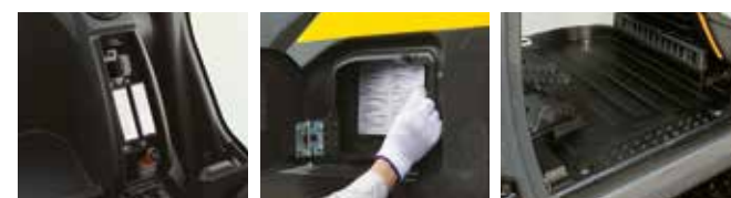
Central fuse box located behind seat
